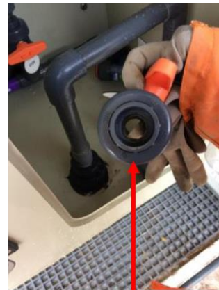
1st inspection of joint indicates lack of glue
