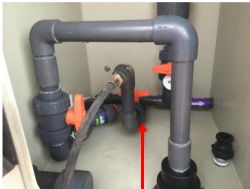
Point of Failure
